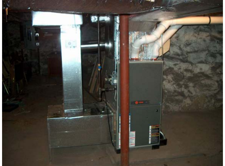
energy efficient heating system – 2003
