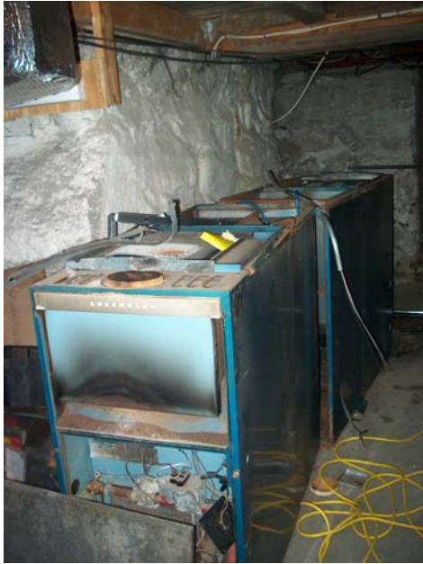
Spalding House – old heating system
